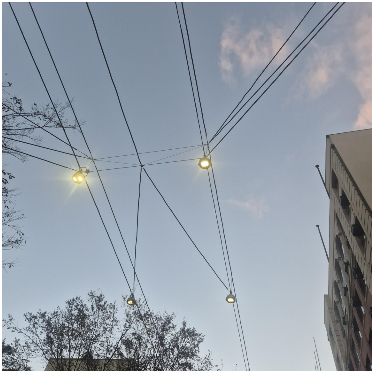
Figure 21. Possum tail covering on Rundle Mall catenary wire
